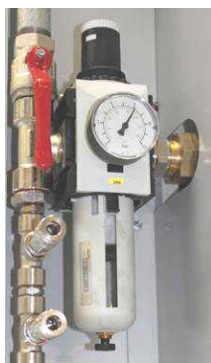
Compressed air supply
