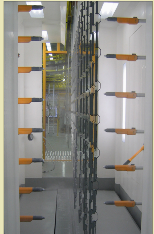
(right) Two fully automated powder coating booths with each 18 automatic guns.
